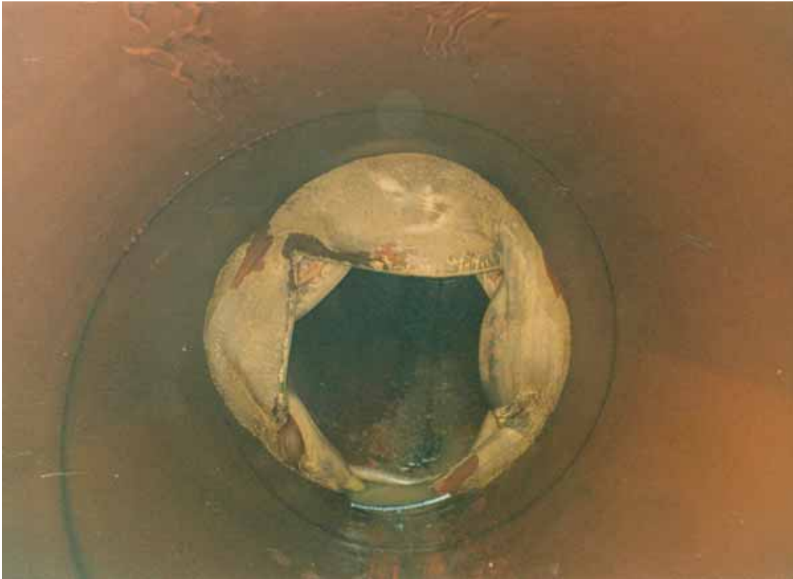
Figure C7-2. Wrinkle of 2.2 Meter Diameter Thames Pipeline
